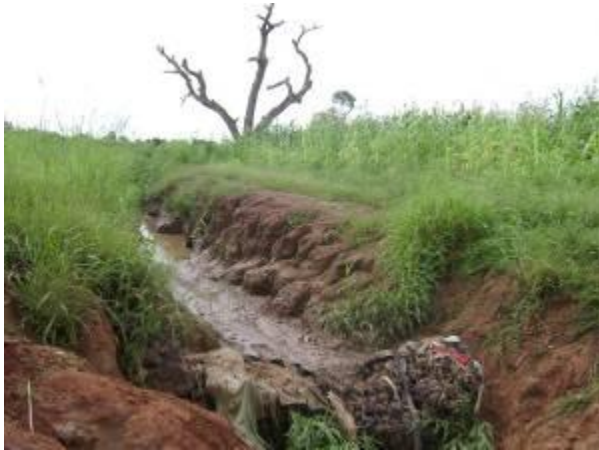
Deposits of sand and other debris accumulating behind a gabion
